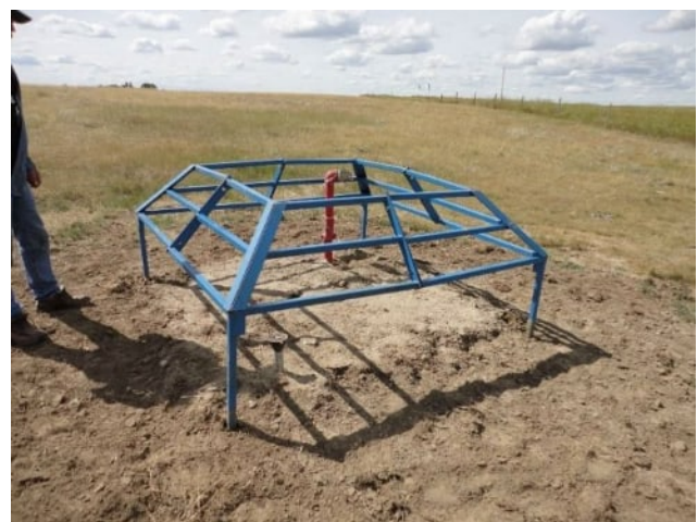
Photo 4: Flushing hydrant and curb stop complete with cattle guard fence
