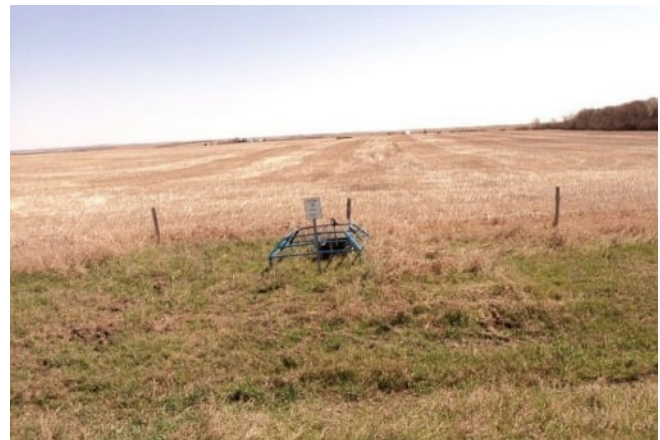
Photo 2: Manual air release hydrant
